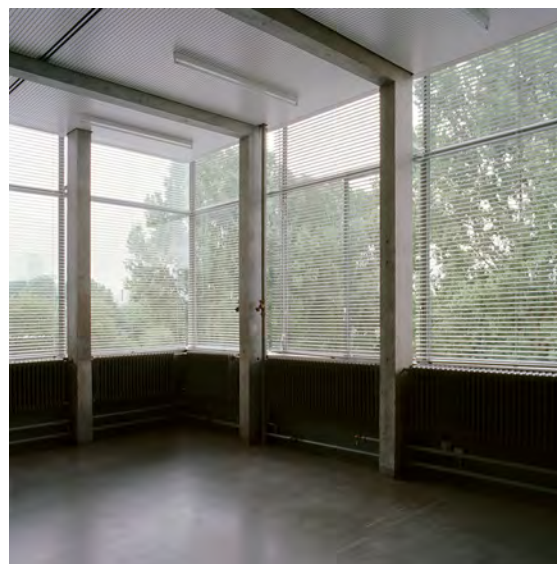
27. Radiators between the columns photo Kim Zwarts (2008)
