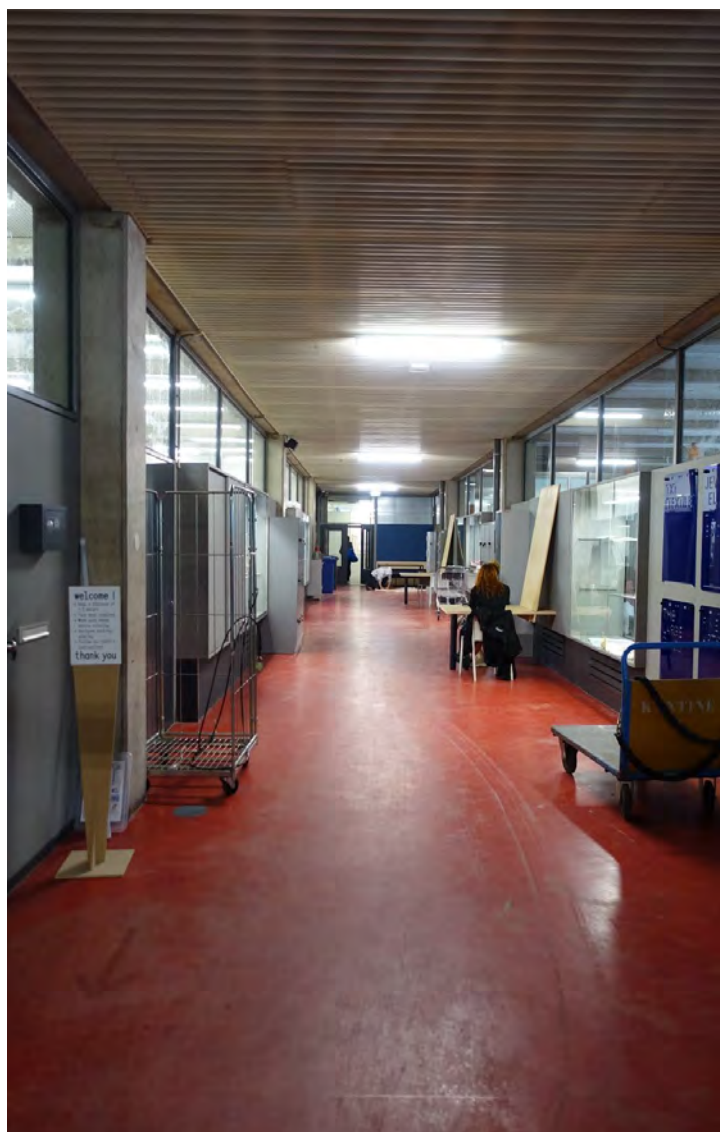
Corridor, ground floor, red Marmoleum floor finish and blue wall, grey walls, dark grey plinths and doors, multi coloured glass cases and cupboards, 2021
